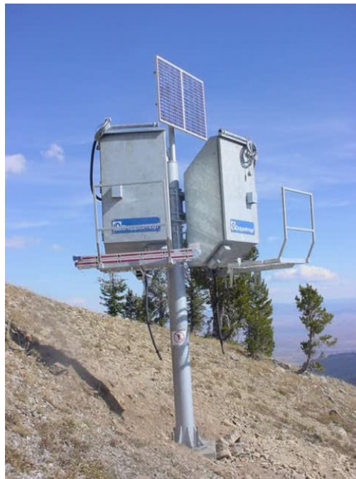
Figure 11 Installed Avalanche Guard system (Rice Jr. et al., n.d.).
