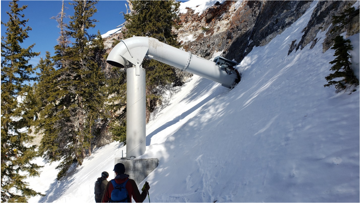
Figure 8 Operational 3.0 m 3 Gazex installed near Alta, Utah.
