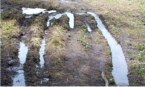
ATV damage Swan Creek Trail. - photo by Phil Knight
