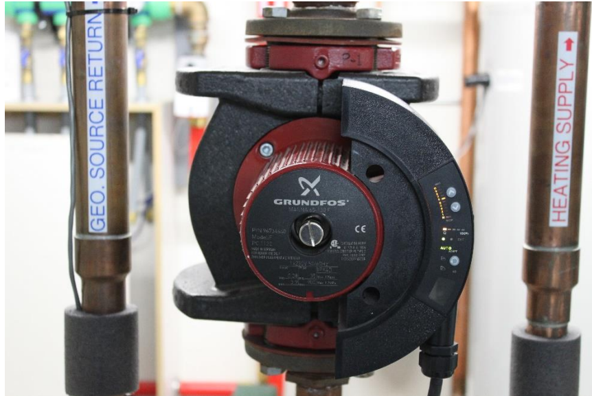
Figure 13. One of the Grundfos® circulators in the mechanical room at the RMEH. They are high efficient electronically controlled variable speed and have different types of automatic settings
