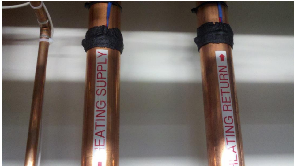
Figure 18. Detail of a pair of type-T thermocouple sensors attached to the copper pipes and covered with asphaltic tape in the mechanical room at the RMEH
