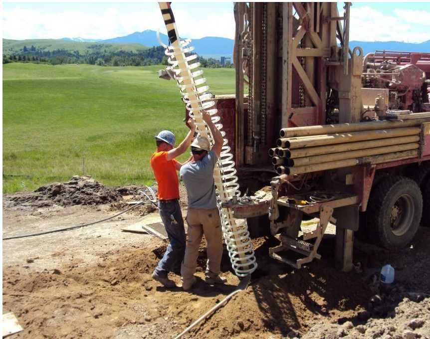
Figure 15. Installation of one the helical GHE at the RMEH
