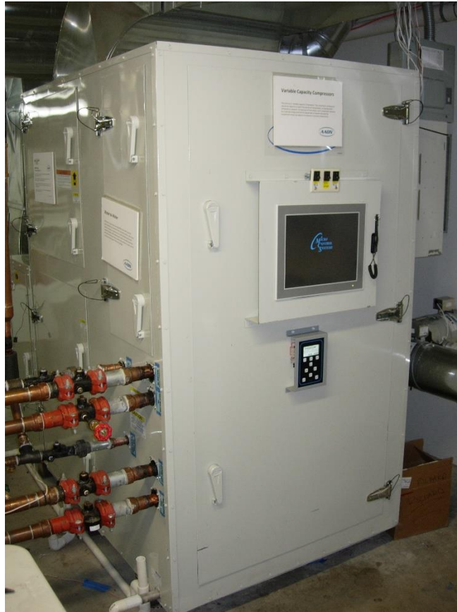
Figure 11. AAON® ground source heat pump in the mechanical room at the RMEH
