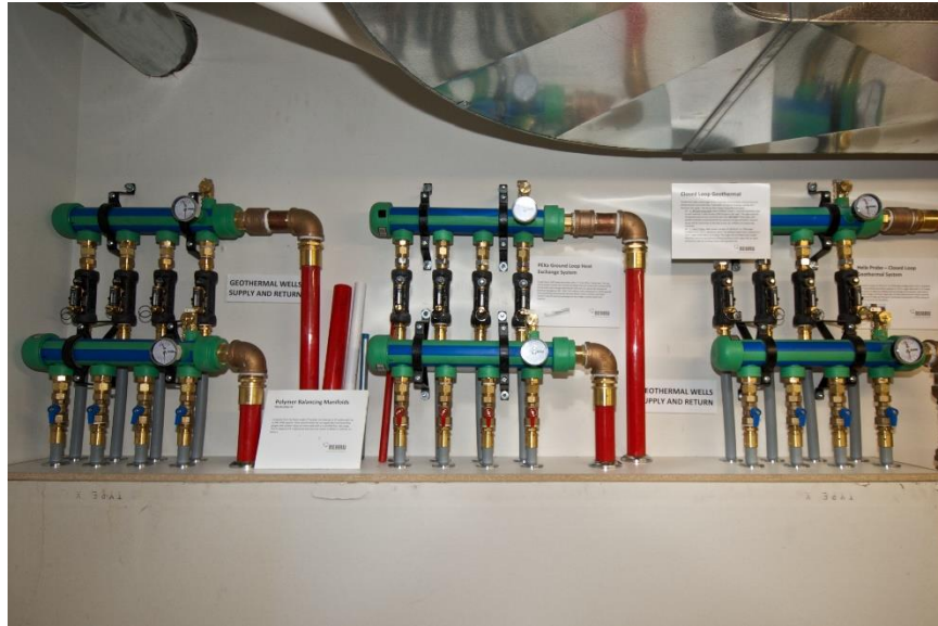
Figure 12. REHAU® PROBALANCE® XP manifolds in the mechanical room at the RMEH are used to distribute and regulate the flow of the geothermal fluid in the ground loops. Headers are made of extruded polypropylene pipe
