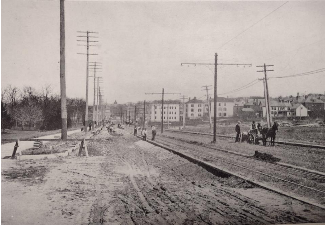
Figure 3.3. Preparation for solid street surfacing on Portland Street (now Park Avenue) between Forest and Deering Avenues, Portland, Maine, 1904. Two carriage lanes, until then gravel and for the moment dirt, were divided by the existing streetcar rails and electrification, which was itself at most eight years old at the time. A smooth sidewalk, likely concrete, is also visible on the edge of Deering Park to the left.
