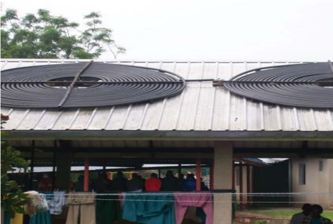
Fig 4.4 Stelehe Orphanage in Tanzania uses locally available black tubing to pre-heat water for washing. This uses solar energy, and saves valuable electricity for other uses
