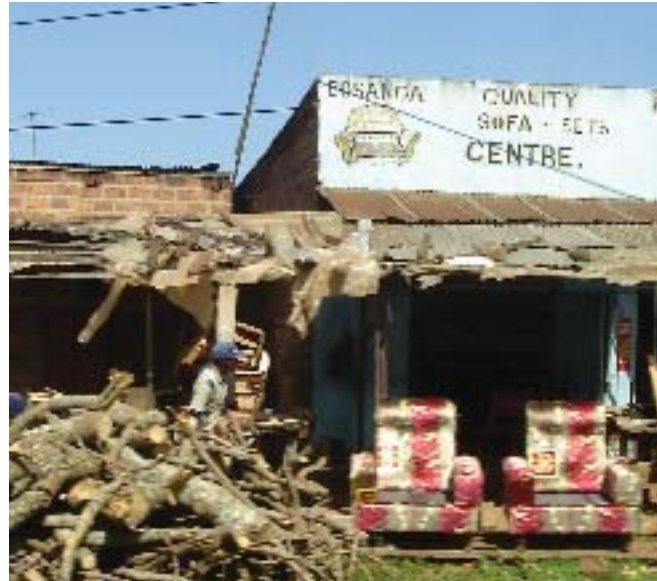
Fig 4.3 A row of shops outside of Mwanza - designed without windows or ventilation. These buildings are relatively new, and are deteriorating
