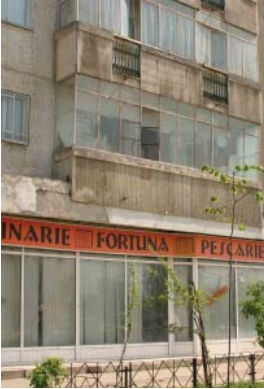
Crumbling buildings in peripheral neighborhoods
