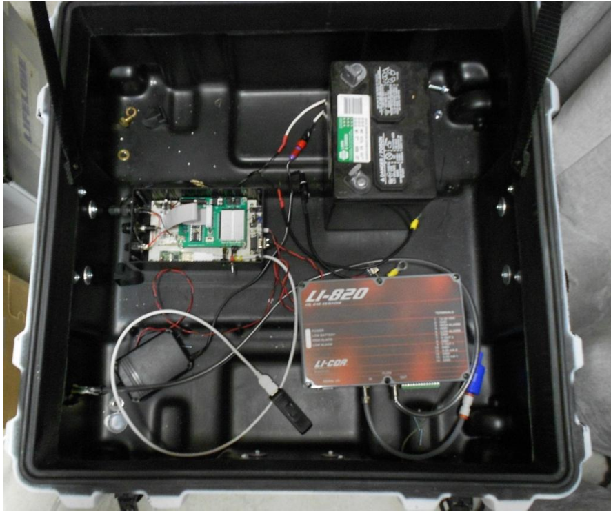
Figure 44: LI-820, data logger circuit and battery all within the weatherproof container used for remote CO 2 measurements
