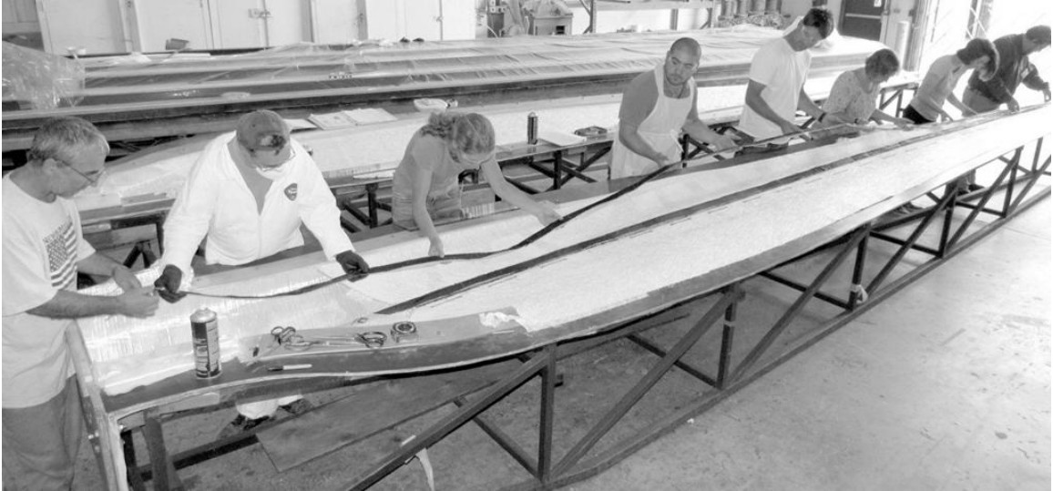
Figure 48: The group effort required to place and align the spar cap without disturbing the IP waves (Rumsey, 2013).
