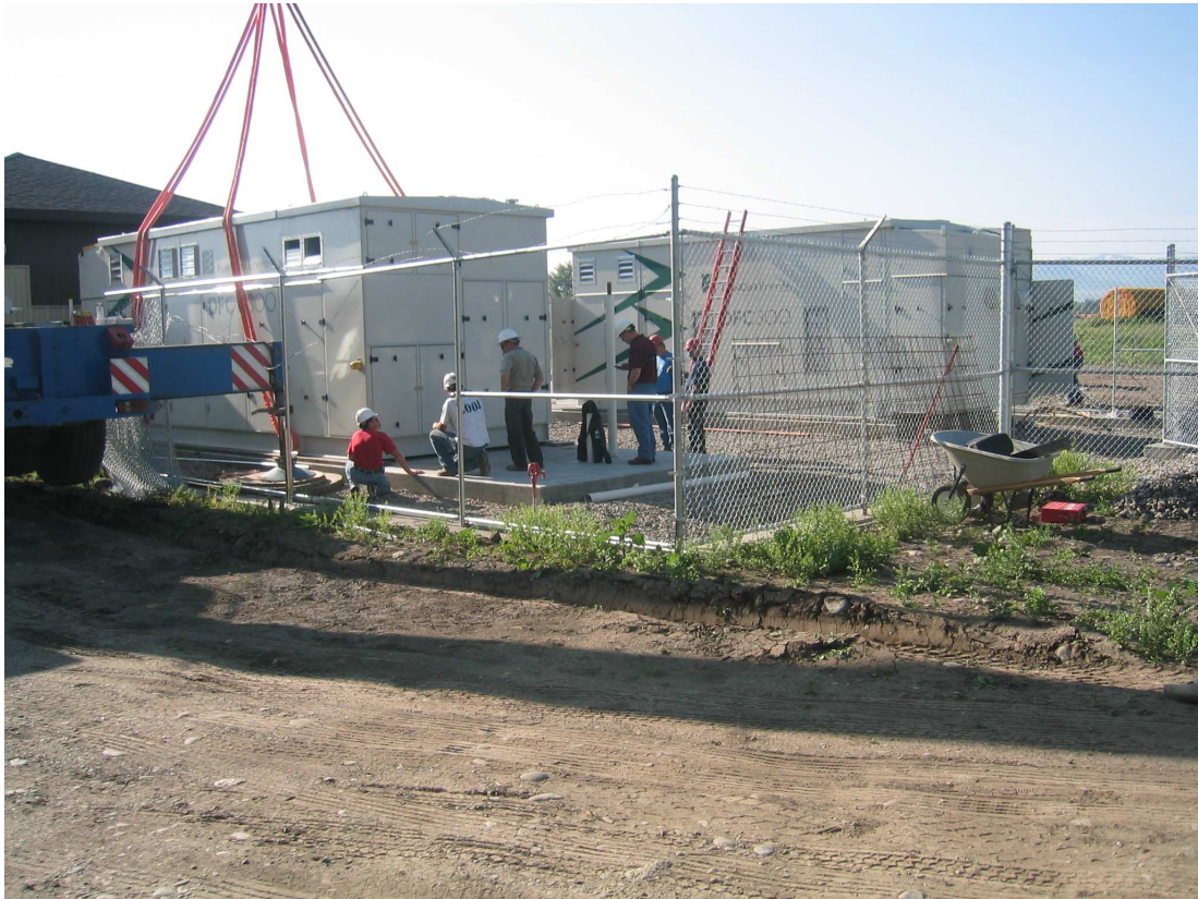
Figure 2: The installation of two FuelCell Energy 250 kW DFC300A molten carbonate fuel cells at Zoot Enterprises.
