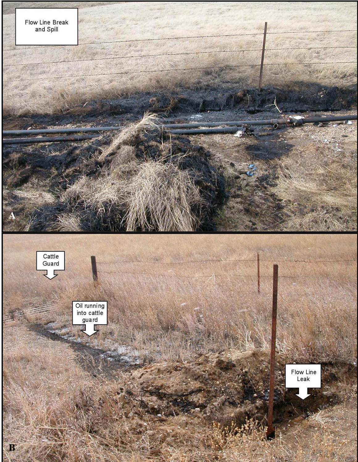
Figure 31. Photo A shows discharged oil and co-produced water from a transport line rupture north of oil field site 126 in March 2006. Photo B shows where oil and co-produced water flowed overland before filling the cattle guard immediately north of oil field site 126 (Photos courtesy of Mickey McCall, SCCD).
