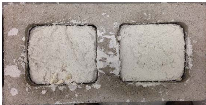
Figure 11. Shrinkage of perlite grout in prism
