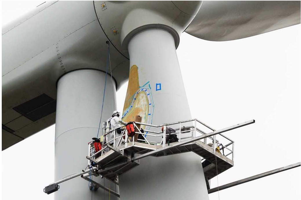
Figure 22. A wind turbine blade technician using a suspended platform to conduct a large repair [1].
