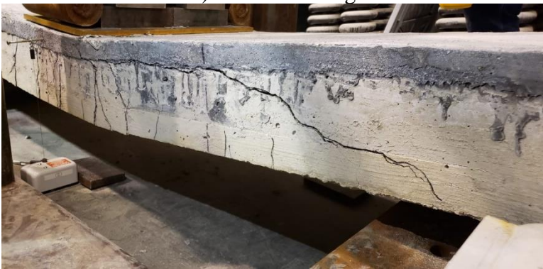
c) Shear crack formation
