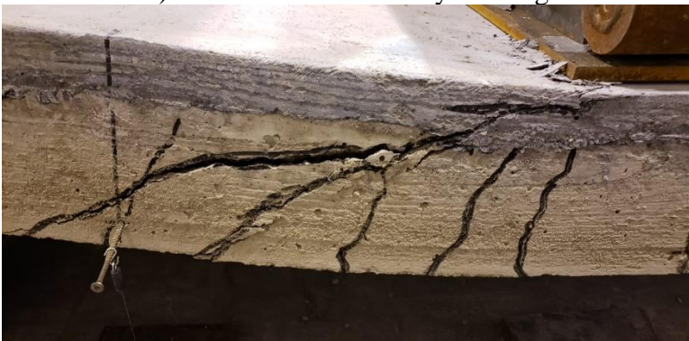
b) Shear crack extending through the overlay
