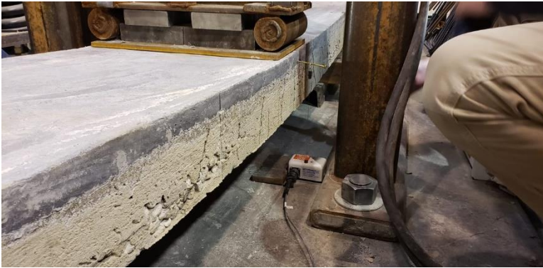
a) Flexural cracks initially forming
