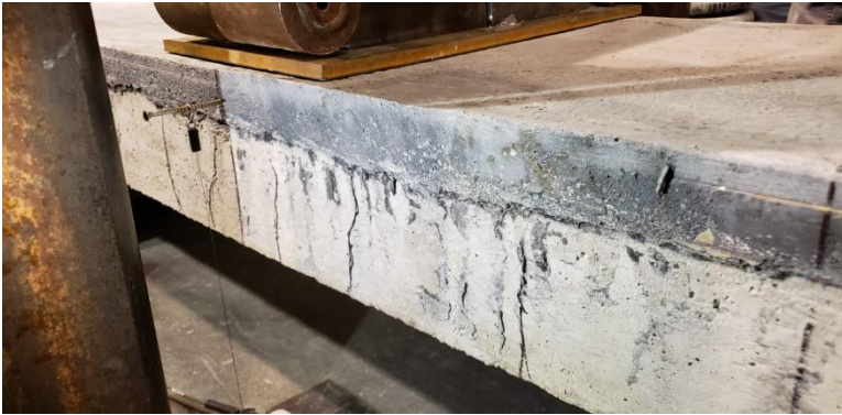
a) Flexural cracks initially forming
