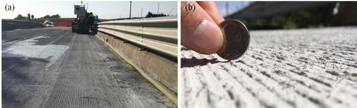
Figure 3: UHPC overlay on Mud Creek Bridge deck: (a) grooving of the surface; (b) closeup of finished surface [23]
