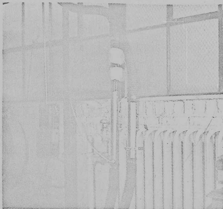
Fig. 10. Picture of Coils and Vent
