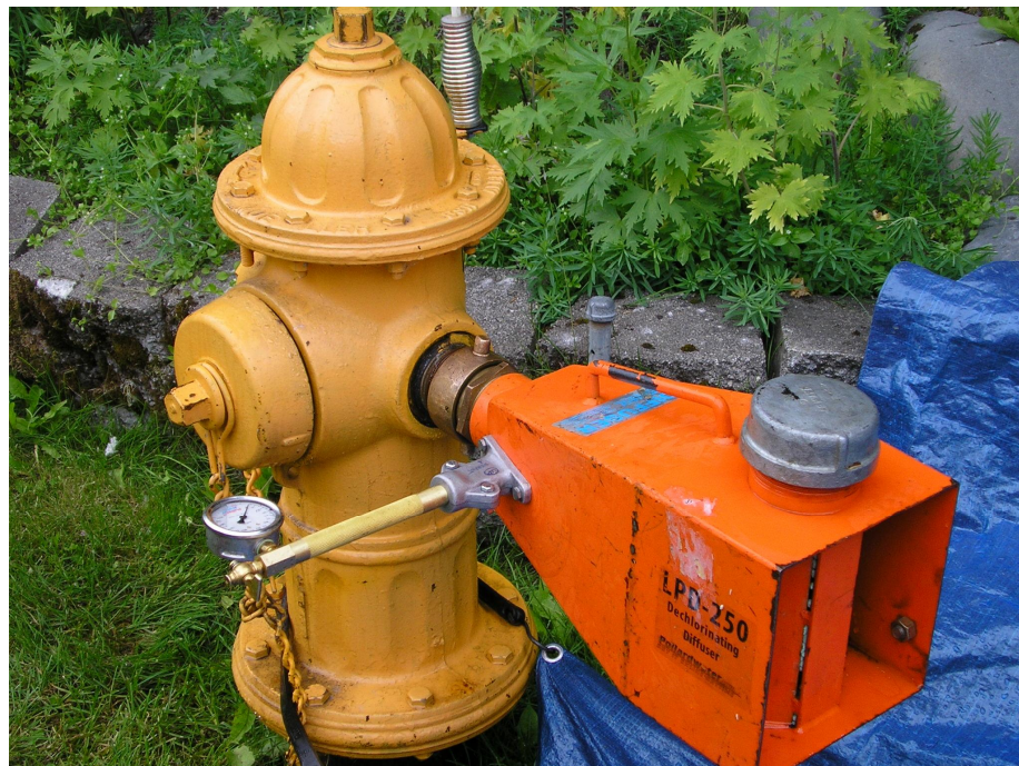
Figure 3.7 Dechlorinating Diffuser with Pitot Gauge Attached
