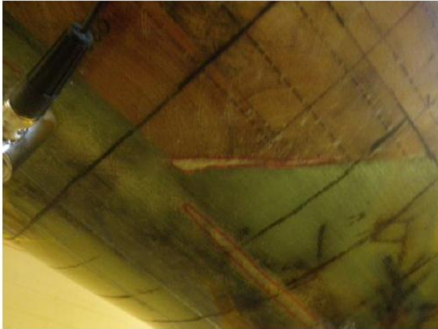
Figure 105: Failure at the 1.2 m location
