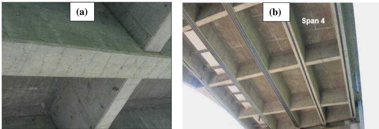
Figure 1. Louisa-Fort Gay bridge, Kentucky; before (a) and after (b) strengthening (Choo et al. 2007).
