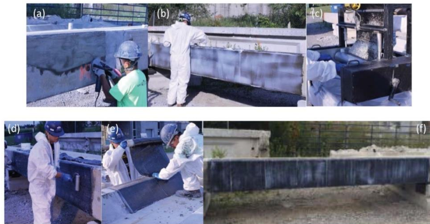
Figure 3. FRP application by wet layup method; surface preparation (a), epoxy application to concrete surface (b), placing FRP to structure surface and epoxy application (c, d, and e) and final FRP strengthened structure (f) (Ghaffary and Moustafa 2020).
