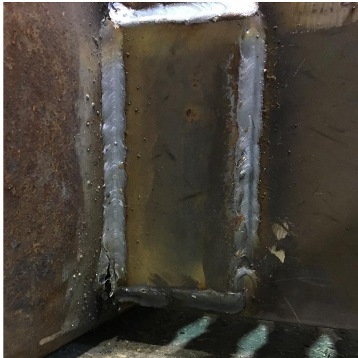
Figure 56 HSS wall buckling failure
