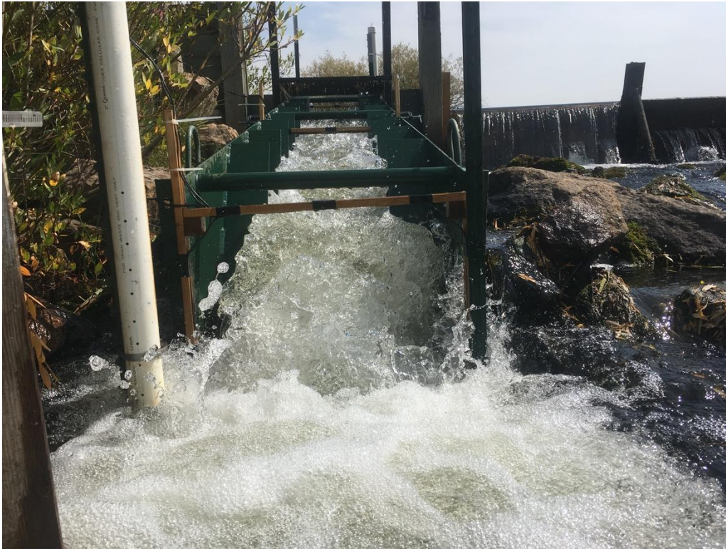
Figure 13: Photo of plunging entrance conditions during Trial 11 on the Big Hole River. The deep upstream depth, steep slope, and shallow downstream depth (Table 1) resulted in a turbulent entrance plunge that appeared to limit entrance of trout and Arctic Grayling during this trial.
