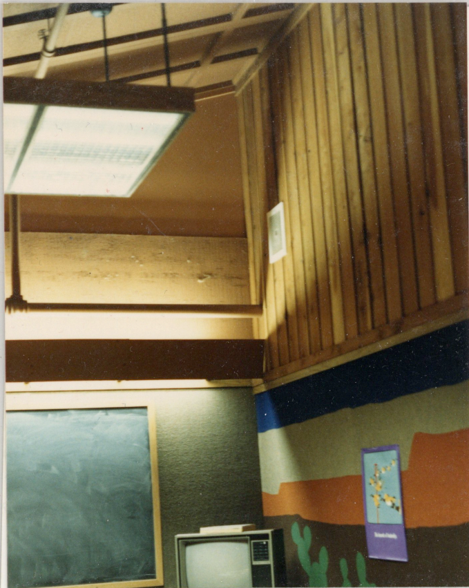
CONFERENCE ROOM WALL SHOWING PANELED ADDITION THAT NOW ALLOWS PRIVATE MEETINGS, BUT PREVENTS AIR CIRCULATION.
