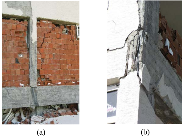
Figure 75: Severely damaged structural elements found in the collapsed school building; (a) masonry exhibiting large shear cracks and crushing, (b) concrete beam-column connection failure as a result of poor detailing (DataHub 2015)
