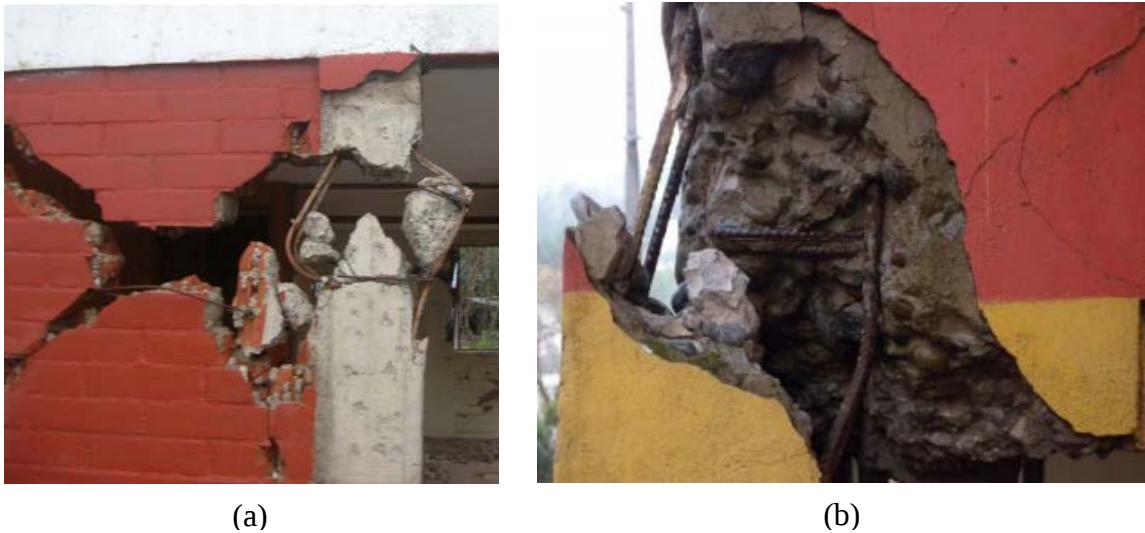
Figure 9: Inadequate reinforcement detailing causing (a) buckling of longitudinal column reinforcement, and (b) shear cracks forming at connection of tie-column and tie-beam (Brzev, Astroza et al. 2010)
