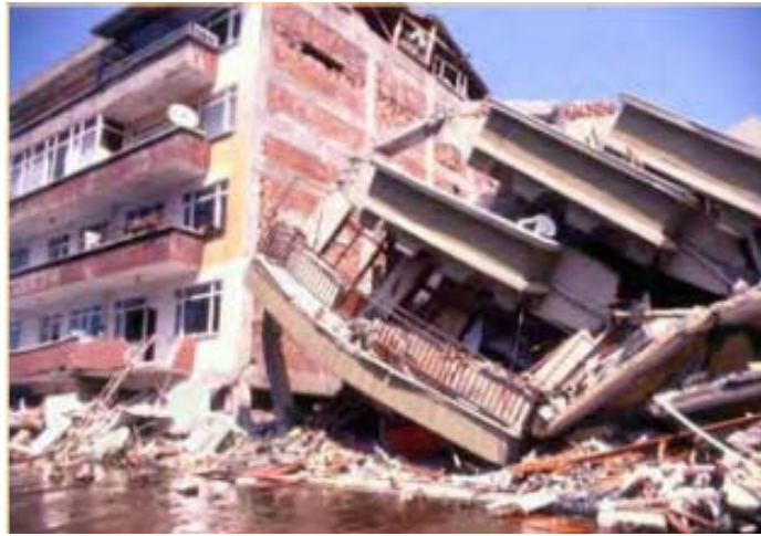
Figure 6: Multi-story collapse due to strong beam-weak column design in 1999 Turkey earthquake (Murty, Brzev et al. 2006)
