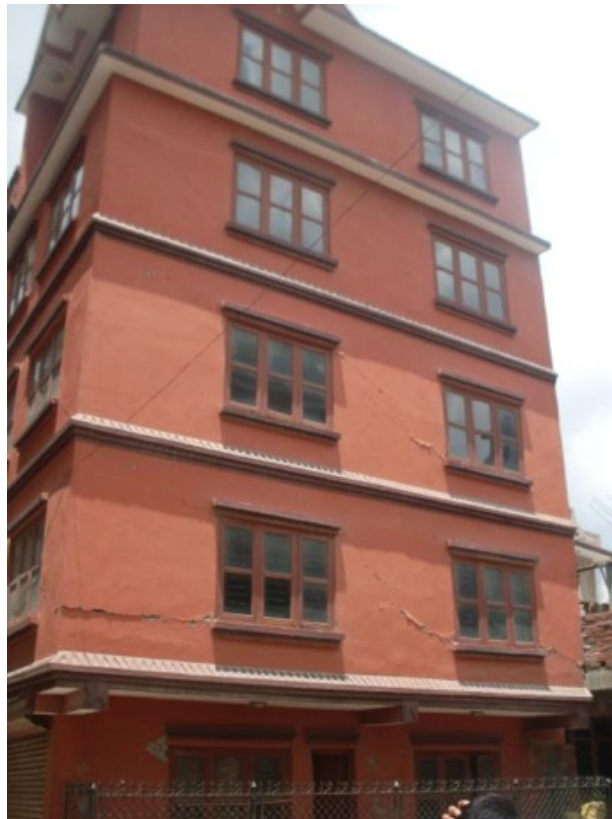
Figure 60: Masonry damage observed on the eastern wall of the Gongabu Bus Park Building 2A
