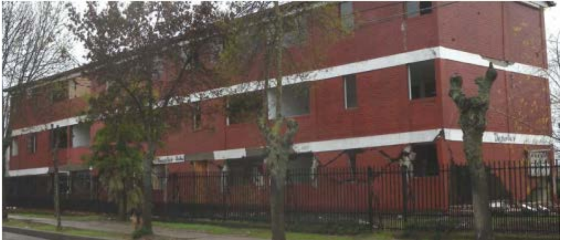
Figure 8: Damage sustained to the first floor of a three-story confined masonry building after Chile's 2010, 8.8 Mw earthquake (Brzev, Astroza et al. 2010)
