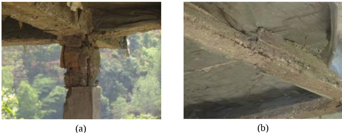
Figure 71: Severe failure caused by poor detailing. (a) insufficient joint reinforcement at beam-column connections, (b) poor quality concrete in structural elements (Lizundia, Shrestha et al. 2016)
