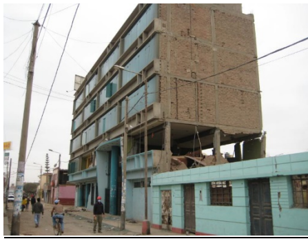
Figure 72: Severely damaged masonry infill building in Peru following the 8.0 Mw earthquake (DataHub 2015)
