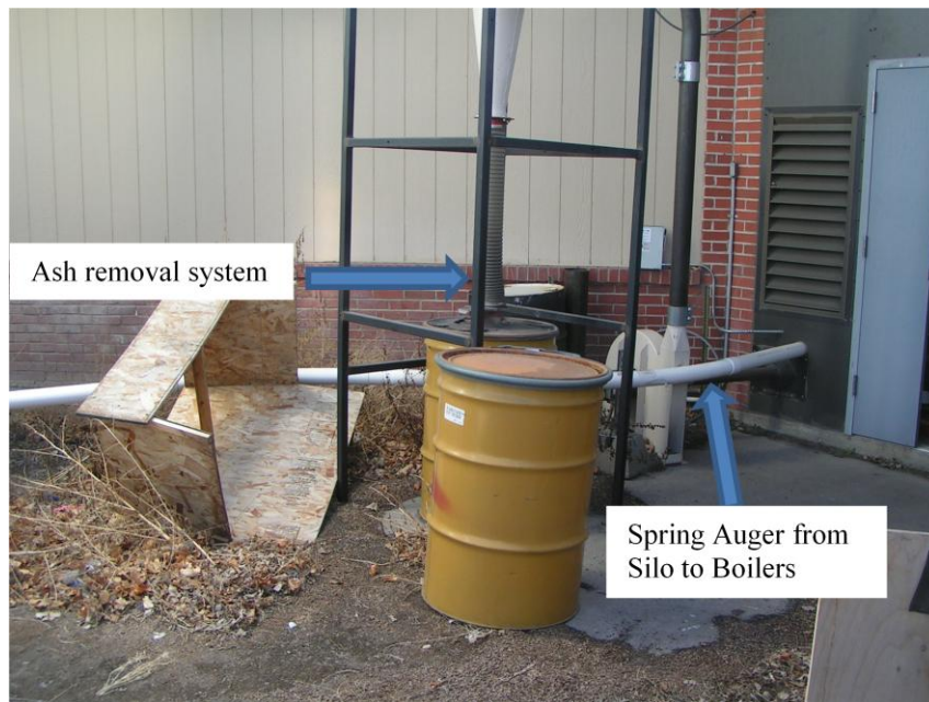
Figure 33: Spring auger and ash removal systems
