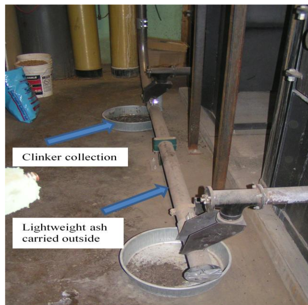
Figure 35: Ash and clinker removal system
