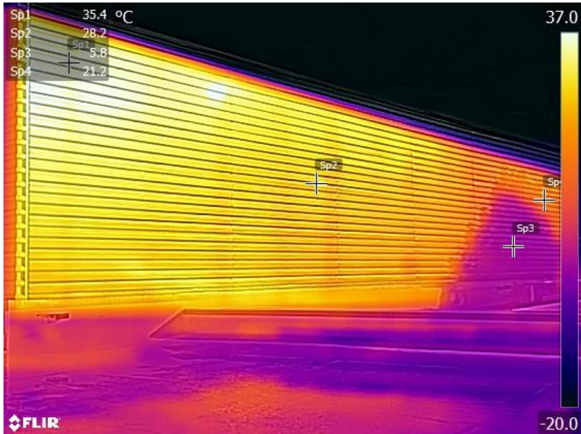
Figure 41: Infrared image of Jab's Hall UTSC 2015/10/23 10:35
