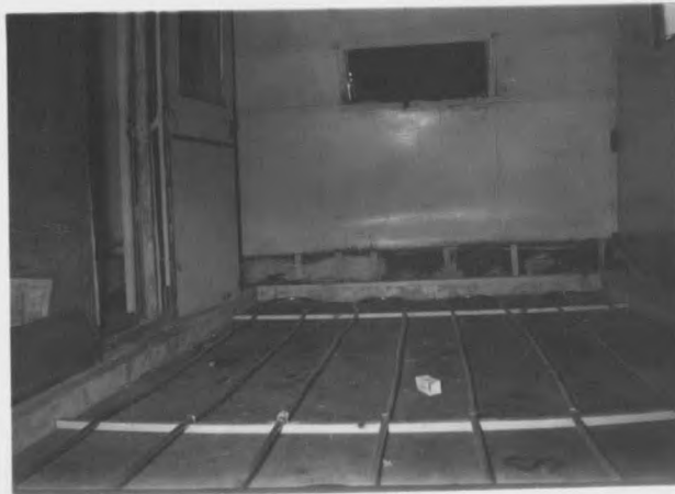
Figure 6 North End Top Panel
