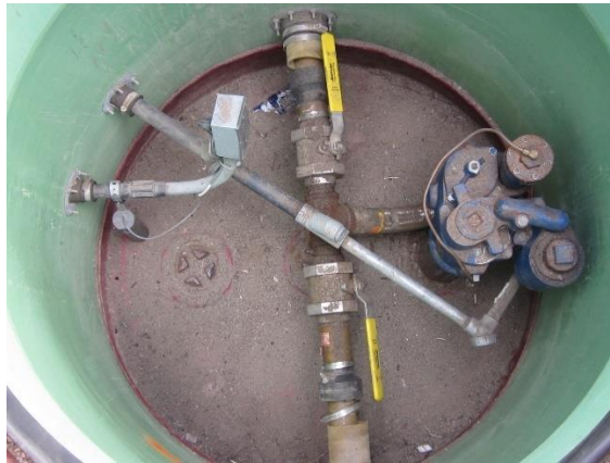
Figure 4. Piping containment sump (Nevada DEP, N.D.).
