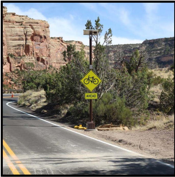
Figure 8. Dynamic Bicycle Detection and Warning System installed at site 1.
