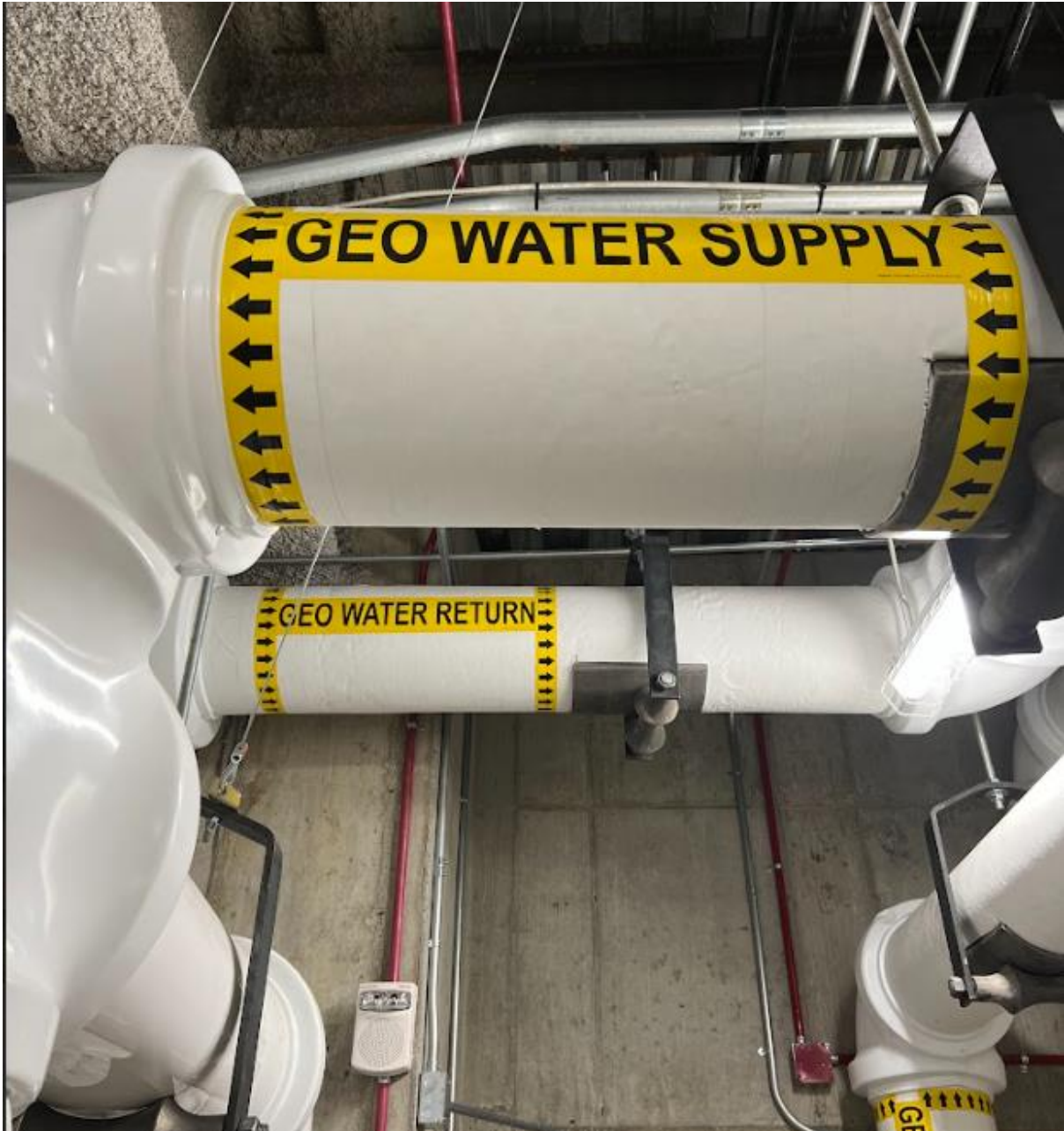
Figure 6. Ground Loop Water Supply and Ground Loop Water Return from Heat Pump Loop System in NAH
