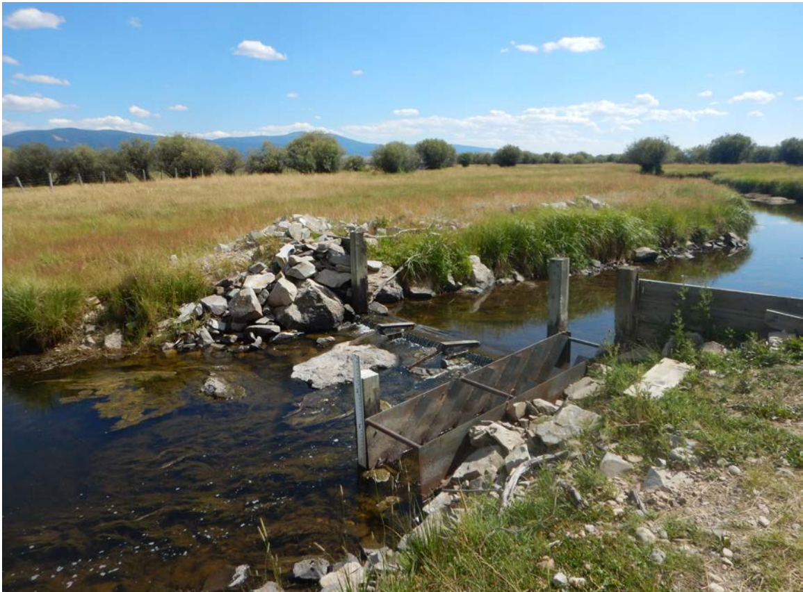
(above) Steel Creek diversion, operated open (no planks inserted), during baseflow conditions. The existing Denil fishway is shown on the river left side of the diversion.
