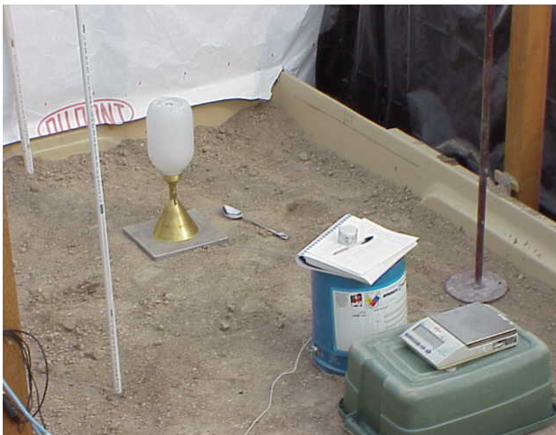
Figure 3.7: Sand cone density tests being performed throughout the backfilling of the soil mass.
