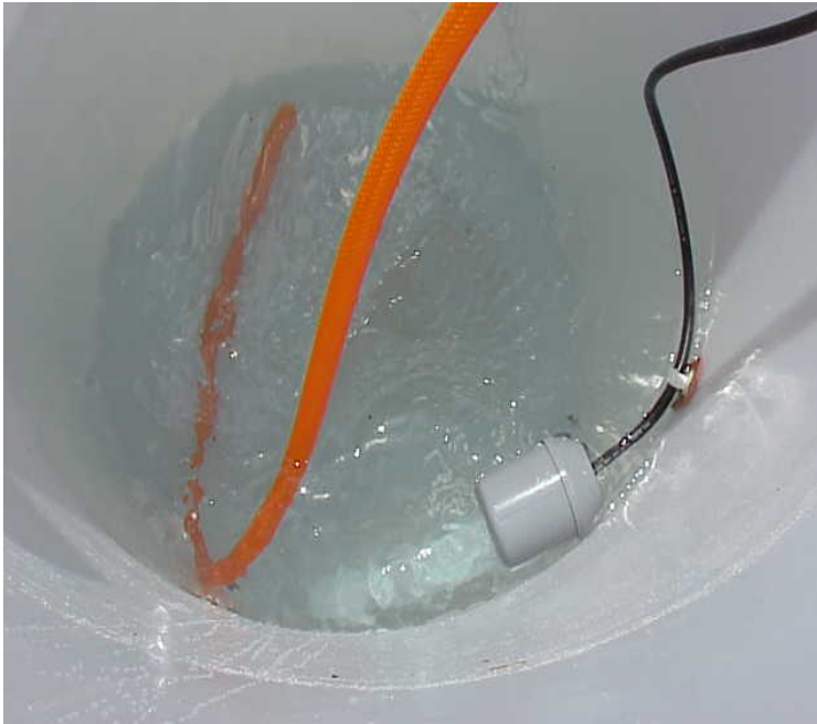
Figure 3.4: Float switch mounted in stock water tank.
