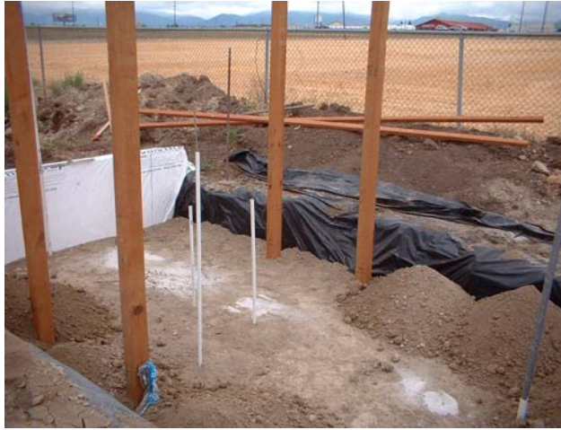
Figure 3.6: Construction of the telltale and reference beams during the backfilling of the soil mass.
