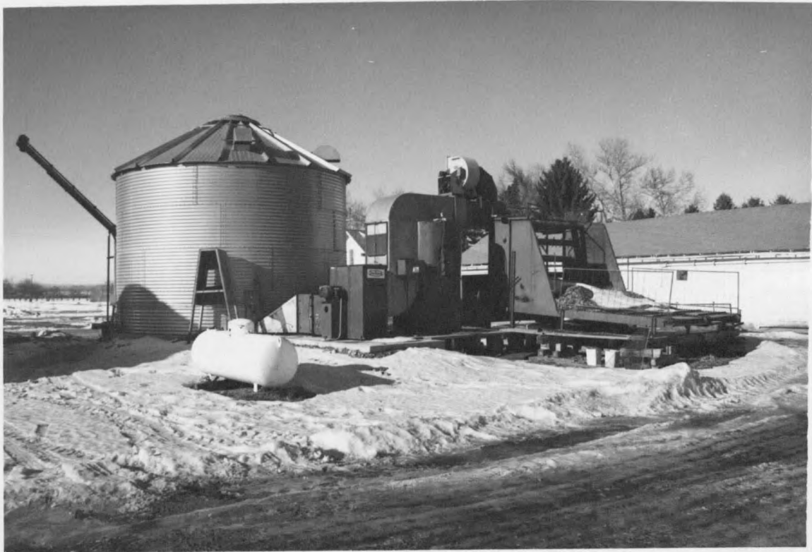
Figure 1. Biomass furnace installation at Huntley, Montana.
