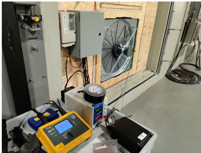
Figure 47. Fan speed control and power measurement instrumentation.
