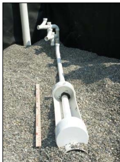
Figure 4: In-cell sample collection tray shown during installation.
