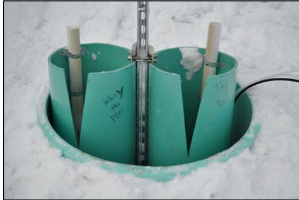
Figure 3: Cell outflow weirs before installation, with infrared sensor mounts attached, but without sensors installed.
