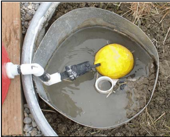
Figure 5. Rojo® valve in stilling well.
