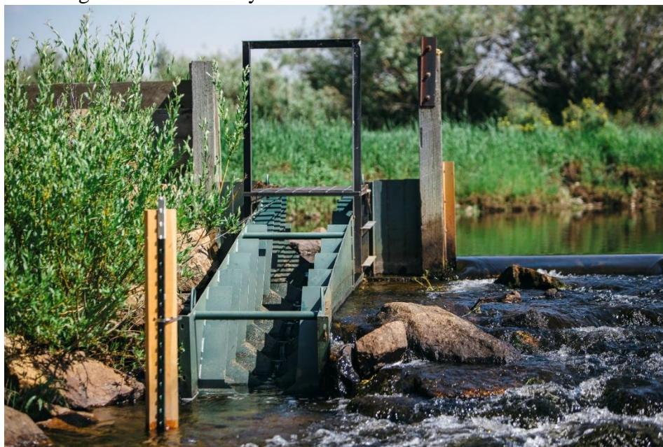
Figure 1: Full scale simple Denil installed at an irrigation diversion and operating during a low flow condition in the Big Hole River Valley.
