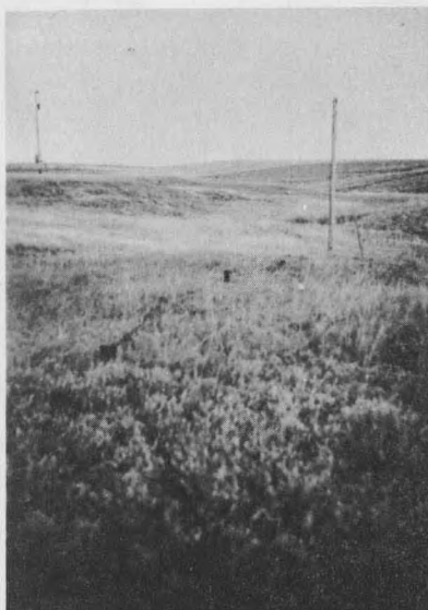
Fig. 16. Ground bed of cathodic protection station shown in Fig. 14. Rectifier cabinet on pole in distance.
