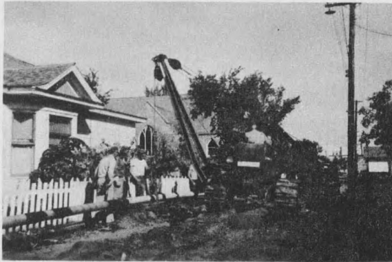
Fig. 1. The cost of corrosion. A 6" gas main no longer serviceable because of leaks, is being replaced by new pipe at left.
