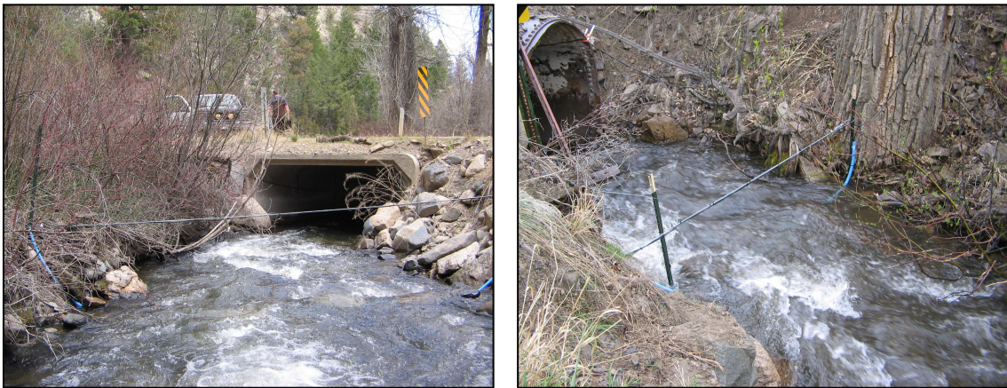
Figure 6. Antenna construction design for the natural control reach and for culverts where the antenna could not be attached directly on the upstream end of the culvert or within the culvert. Left: inlet of culvert 3. Right: inlet of culvert 5. The lower portion of the antenna loop is encased in the plastic conduit and buried in the substrate.
