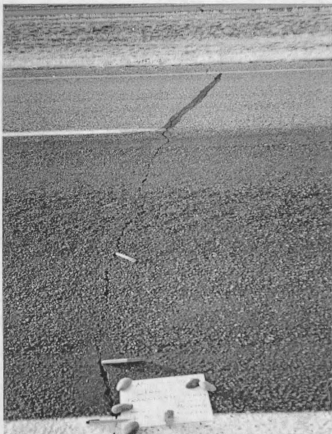
Figure 1. Pre-construction pavement condition.
